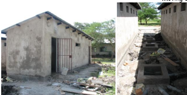
Muungano Secondary School toilets
